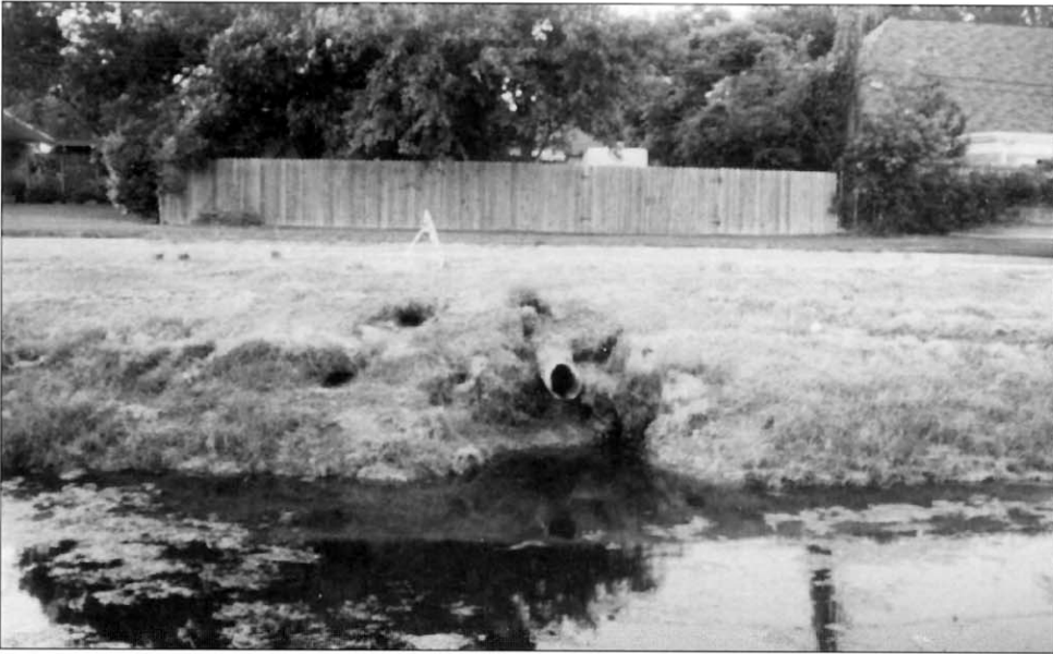
Bank erosion caused by a nutria burrow. Because roadways run parallel to canals in much of Jefferson Parish, nutria burrows sometimes extend underneath the road. If not filled in, these burrows will cause erosion that can weaken the road bed. (Photo by Ryan Almerico)
