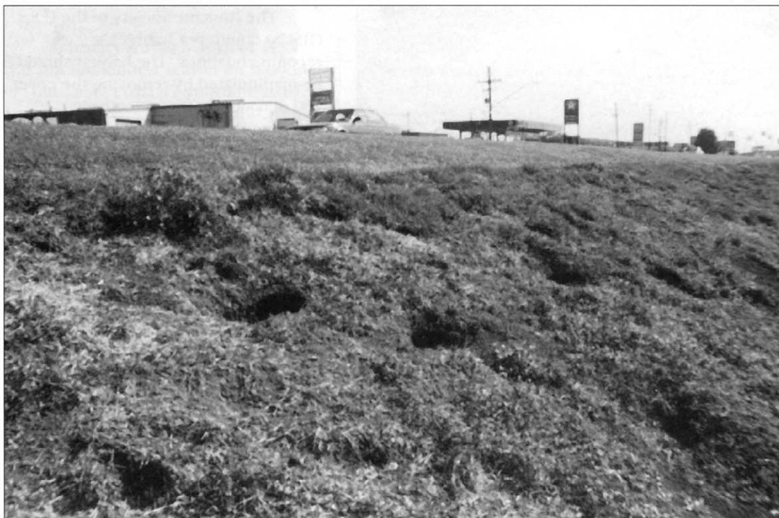
Multiple nutria burrows along Veterans Blvd. Underground, these burrows form a honeycomb of tunnels that weaken roadbanks and make them more likely to cave in. (Photo by Ryan Almerico)
